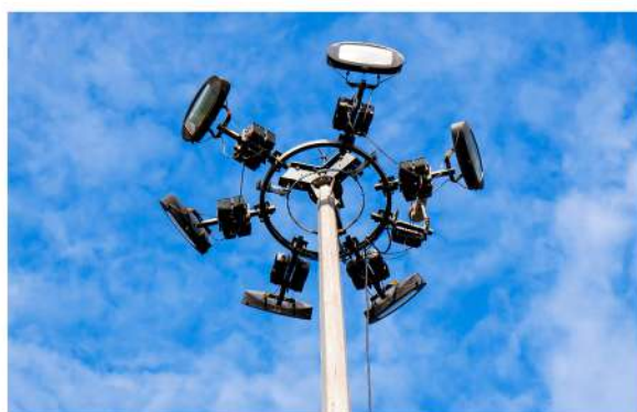
High Mast Light Tower
